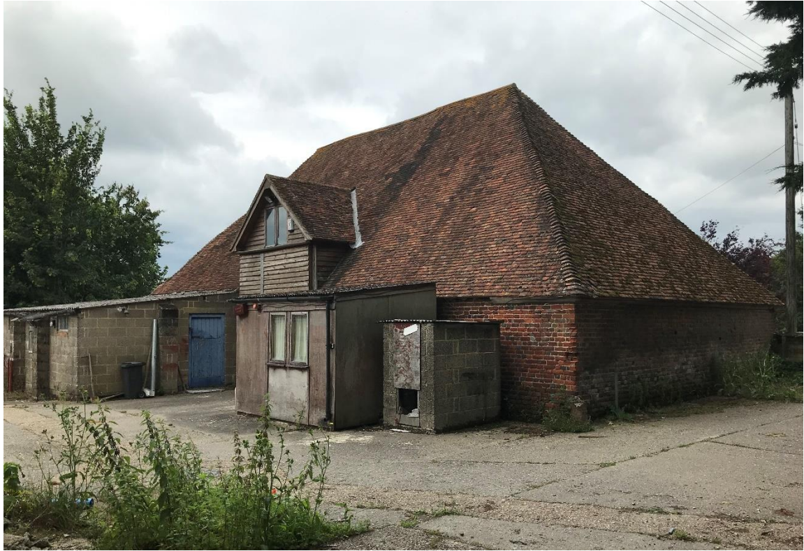
Figure 20: View of Barham Court Farm Barn from the south east (the Site).
