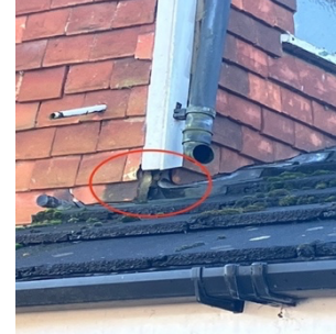
PHOTO 4: Gap into lead flashing corner of building (circled).
