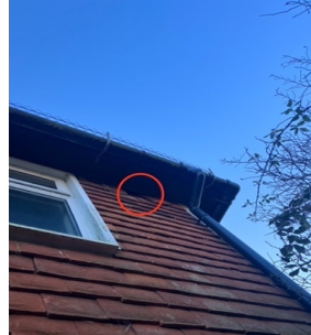
PHOTO 3: Missing tile to the south back corner of the building.
