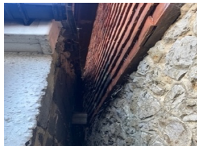
PHOTO 6: Gap between the extension and main walls of building.
