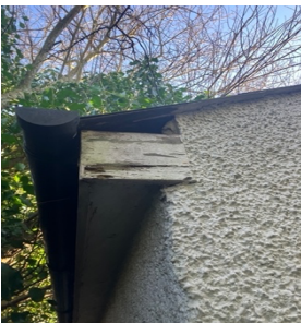
PHOTO 13: Gap between barge board and soffit.
