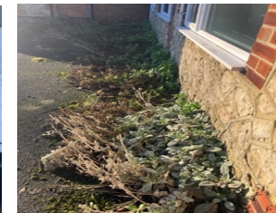
PHOTO 12: Vegetation flush to the east (front) of the building.
