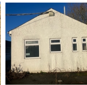
PHOTO 16: East section of the building with gaps under gable point.
