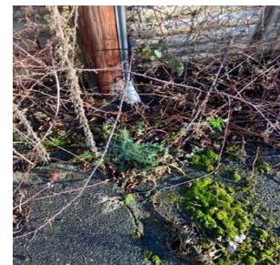
PHOTO 28: Hardstanding and vegetation growth next to north fence.
