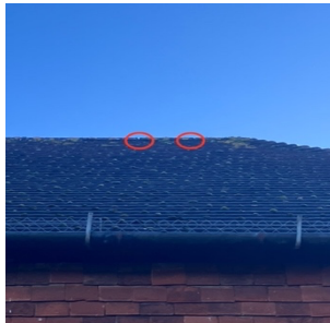
PHOTO 14: Broken ridge tiles (circled) on top of the building.
