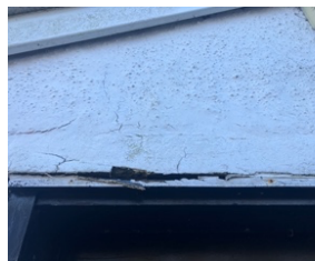
PHOTO 11: Wear and tear gap to the back of building.
